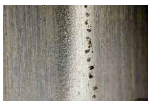
Excessive voltage Sparking and localized heating from current passage in the contact area because of ineffective insulation.
