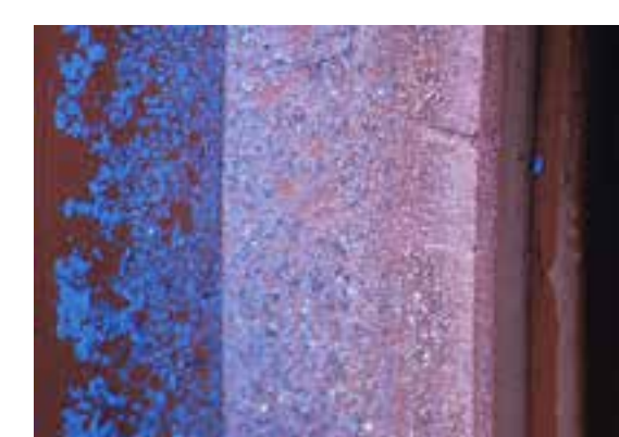
Contamination Paint overspray (blue) introducing contamination and cut lip due to sharp keyway.
