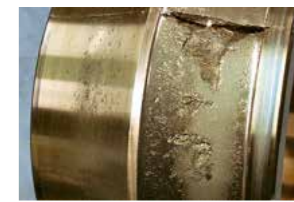
Fatigue fracture A fracture resulting from frequently exceeding the fatigue strength limit of the material.
